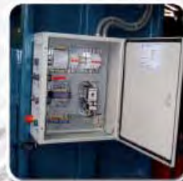
Panel de Control
